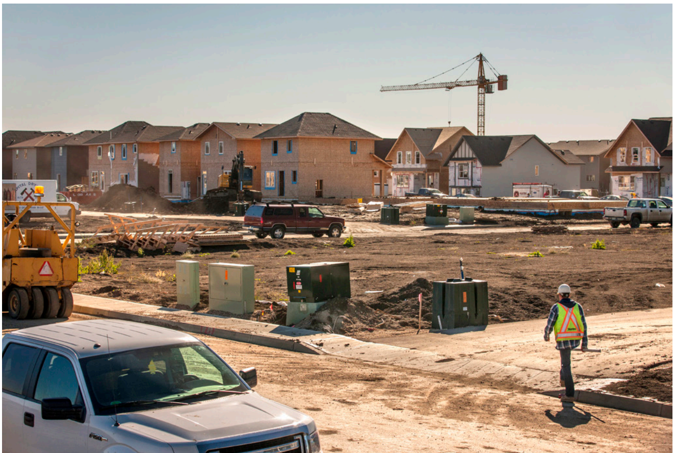
The new Turnkey Solution initiative is continuing implementation. In 2013, it resulted in five major developers taking responsibility for the engineering, materials procurement and installation of Crown distribution infrastructure for 650 residential lots.
