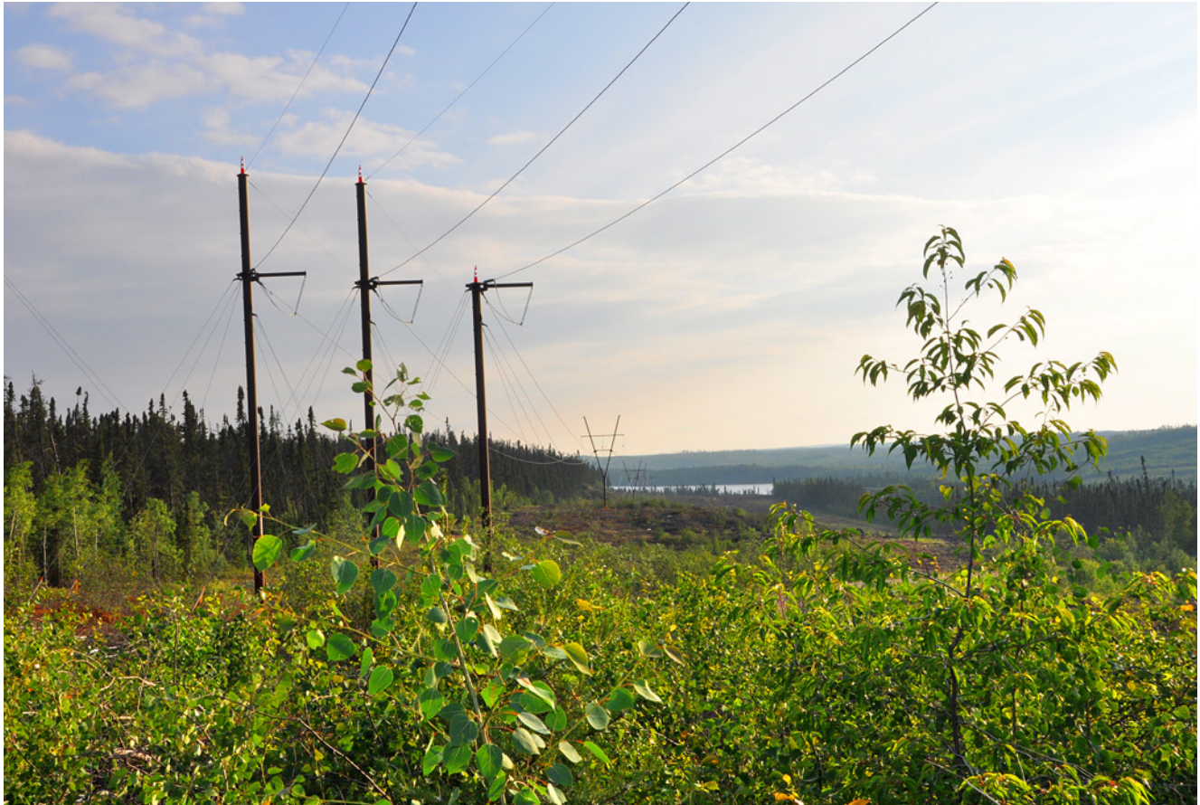
The new $380-million 11K Transmission Line will connect SaskPower's Island Falls Hydroelectric Station to the new Key Lake Switching Station in Saskatchewan's North. The line will improve reliability and accommodate increased electricity demand.
