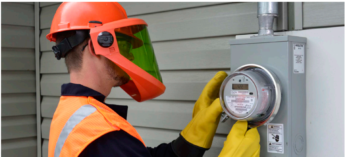
In 2013, we began full deployment of Advanced Metering Infrastructure by installing the first 39,000 of approximately 500,000 smart meters. Future benefits include automatic meter readings that largely eliminate billing based on estimates; faster service connects and disconnects; and quicker identification and tracking of power outages once supporting technology is in place.
