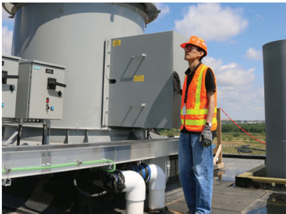
DURING THE YEAR, SASKPOWER COMPLETED A DECOMMISSIONING AND RECLAMATION PLAN FOR THE QUEEN ELIZABETH POWER STATION (PICTURED).
